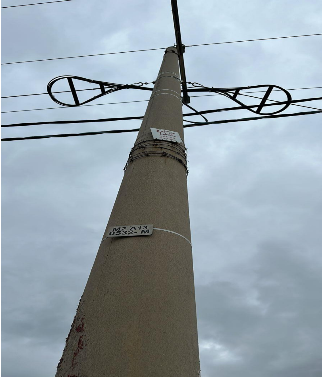
Figure_8 - Aerial Cable Storag
